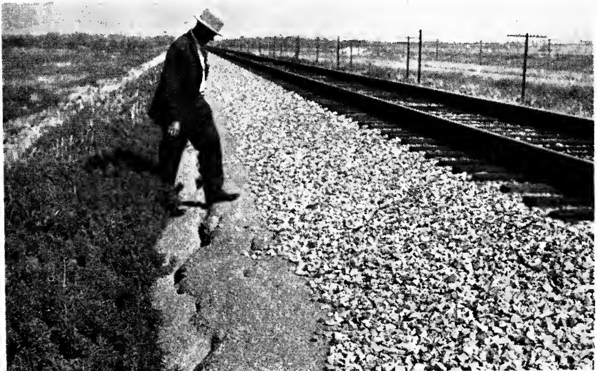
Fig. 5—Fort Gibson revision, open cracks developed during dry season.
